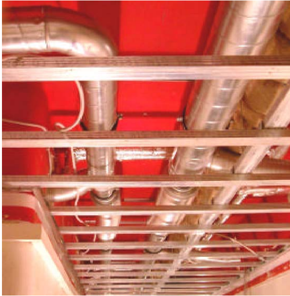
Fig. 5: Ventilation pipes in the ceiling area of the hallways
