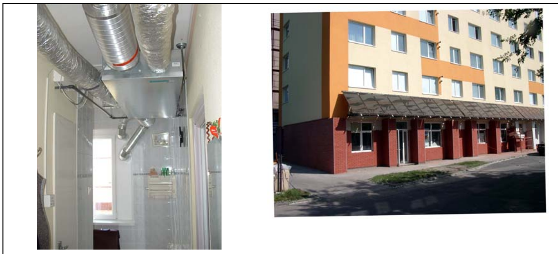
Figure 8: Installed ventilation heat recovery units under the ceiling of the hall. Now they are covered with gypsum board suspended ceiling. Figure 9: Installed solar collector field on the southern side covered with gypsum board suspended ceiling.
