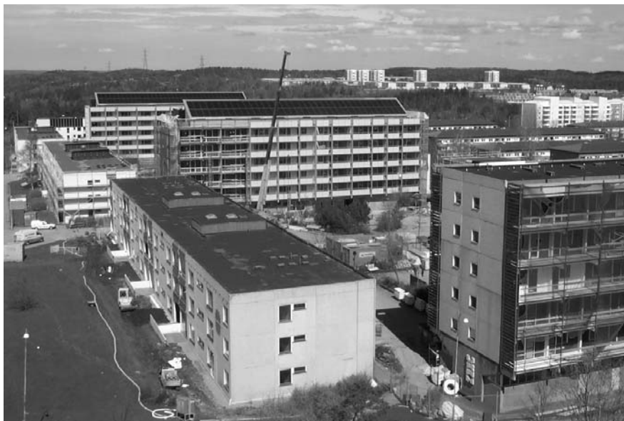
Fig. 11 Overview of all three blocks. The most northern block is finished, the second block is partly ready and the renovation has just started in the third block (closest). Photo: C. Nordström
