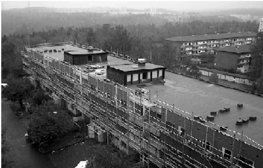
Fig. 10 Low-rise building with new roof covers and enlarged roof tops for the new ventilation systems.
