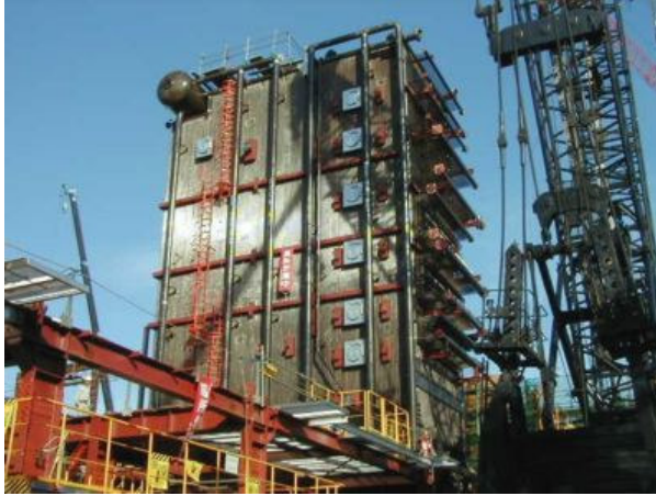
Waste Heat Recovery Boiler for Waste Incineration (Source: IMEX)
