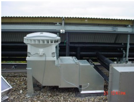
Heat exchanger on roof
